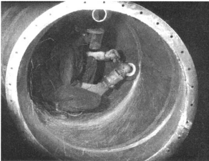
Figure 4.2 Grinding of weld seams in a duct before shot blasting and coating of adhesive.
